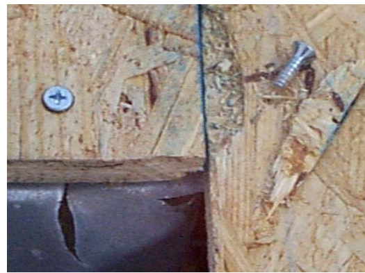
Figure 22- Fatigue failure of sheathing
