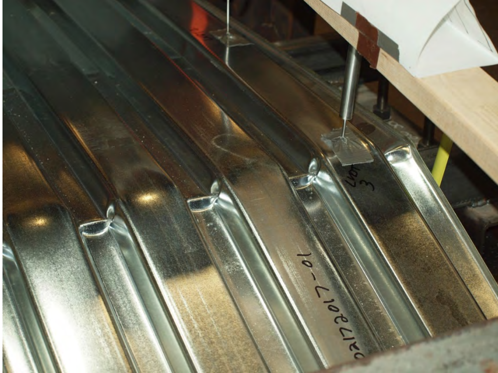
Figure 40: 18 Gage Deck Negative Bending - Further Buckling.
