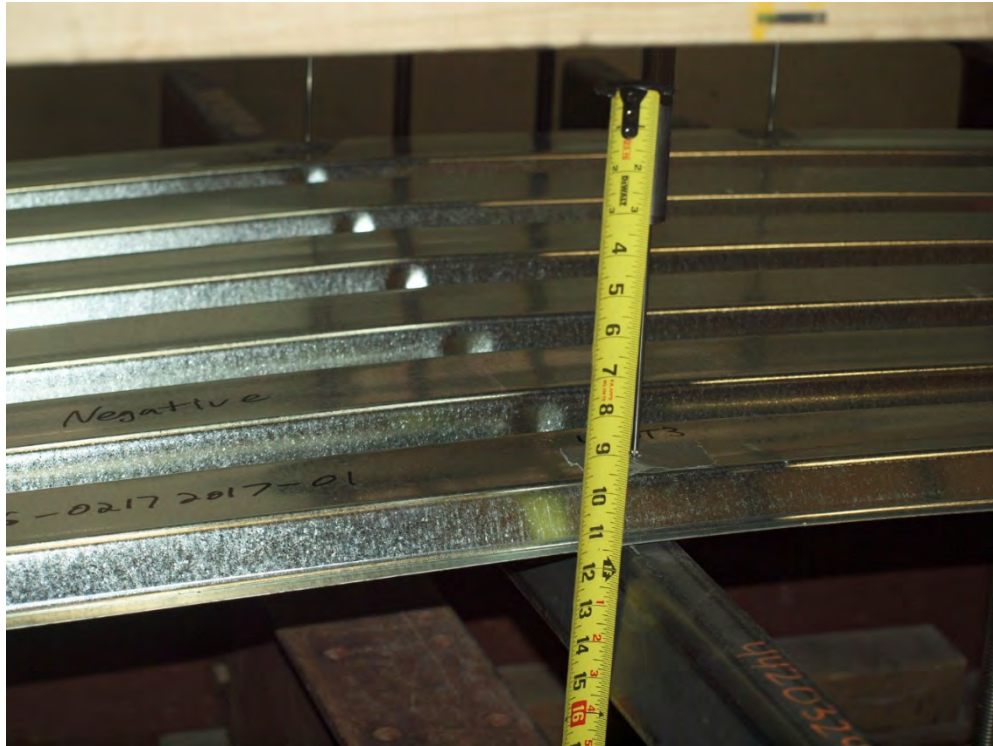
Figure 53: 20 Gage Deck Negative Bending - Initial Buckling.
