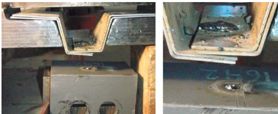
Figure 1.6: Tension weld failure (Guenfoud, 2010).
